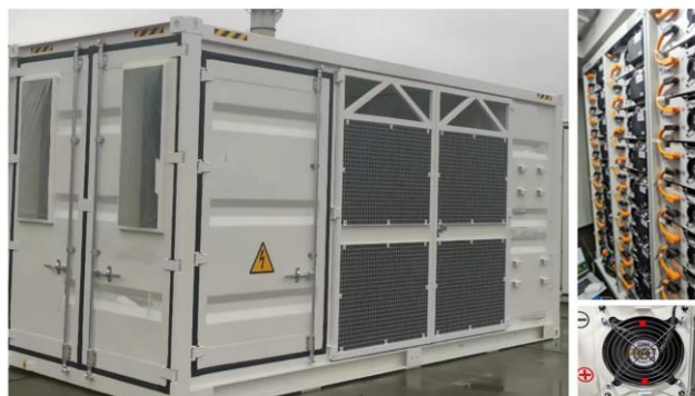
Figure 1. Stadium power supply electric container and internal battery arrays.
