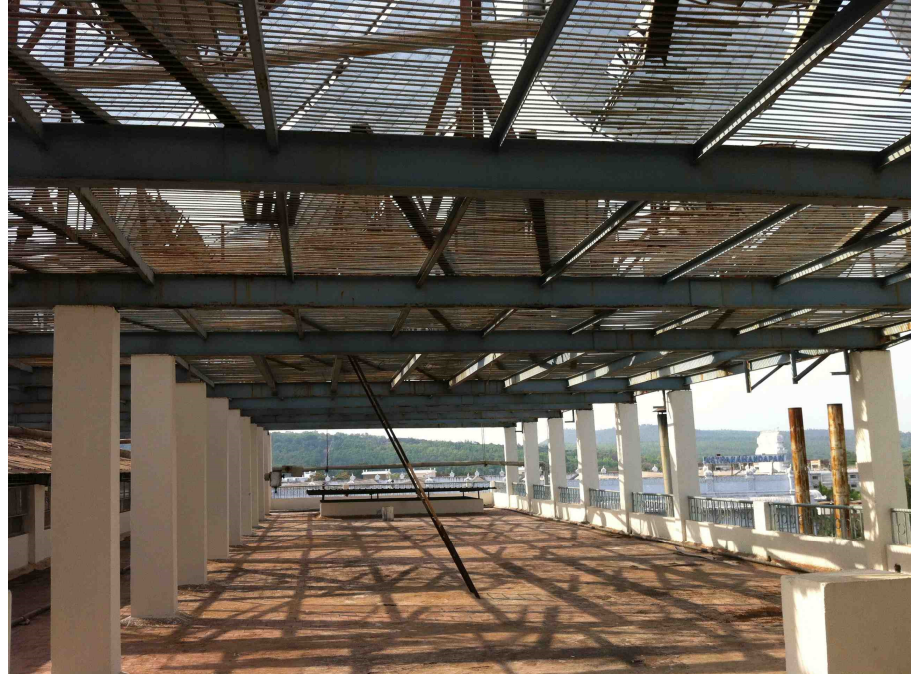
Figure 7. An example of an additional rooftop structure at the Tirupati temple Scheffler Dish installation for cooking food. Photograph by the primary author.
