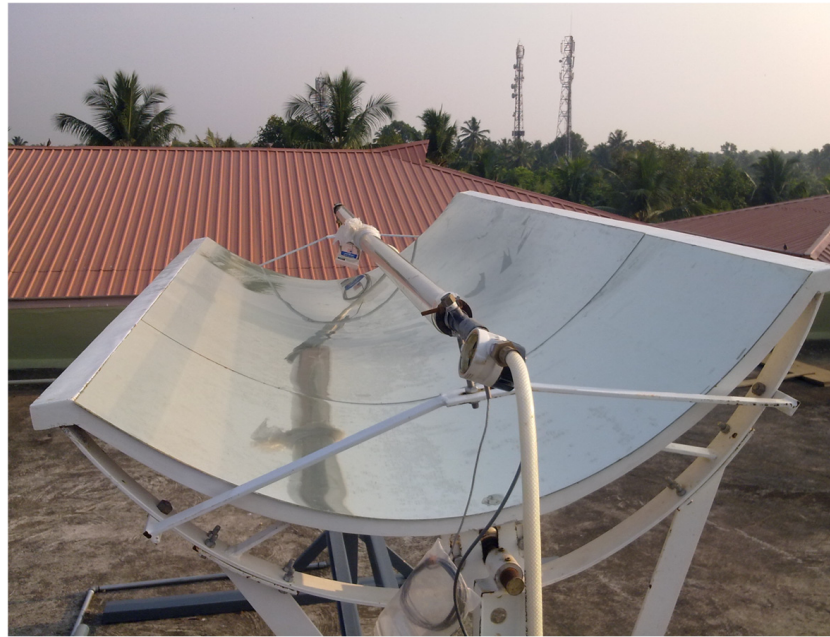
Figure 2. Rooftop-scale parabolic trough. Photograph by primary author.
