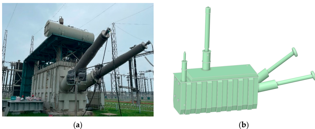
Figure 1. Models of the \pm 400 \text{ kV} converter transformer. (a) Actual geometric model; (b) simulation geometric model.
