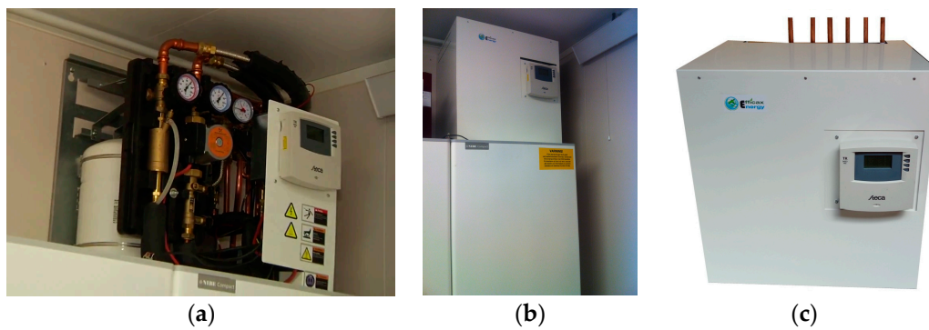
Figure 5. Picture of the prototype: (a) without the external cover; (b) with the external cover; (c) showing the connections to: collector inlet, collector outlet, cold water main, domestic hot water supply to user, auxiliary heater inlet and outlet.
