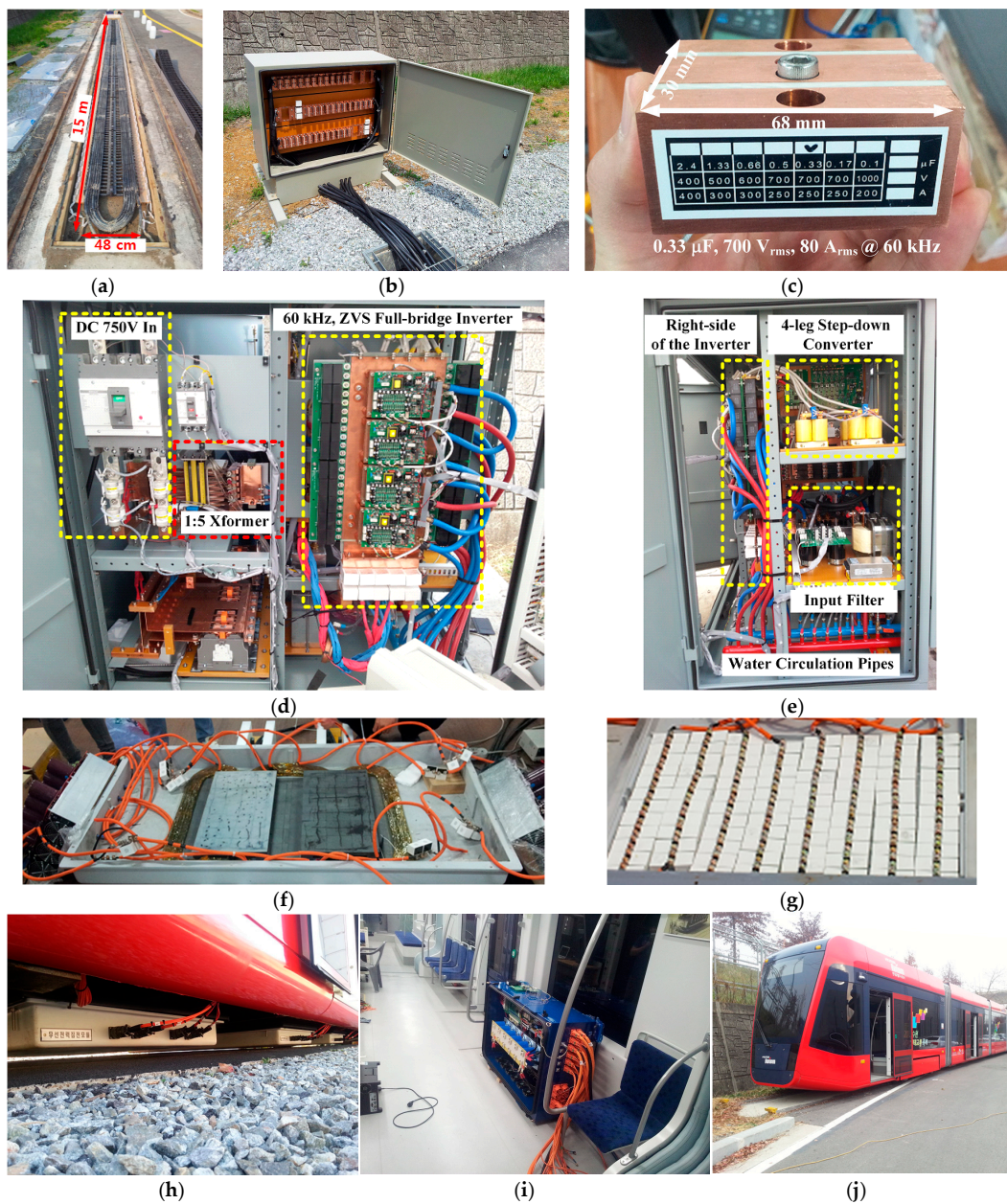
Figure 10. Photographs of the developed test-bed: (a) transmitter; (b) transmitter tuning capacitor bank; (c) transmitter tuning capacitor; (d) the PAM inverter; (e) interleaved DC-DC converter; (f) pick-up winding; (g) pick-up tuning capacitors; (h) installed three pick-ups; (i) pick-up output voltage regulator; and (j) target tram.
