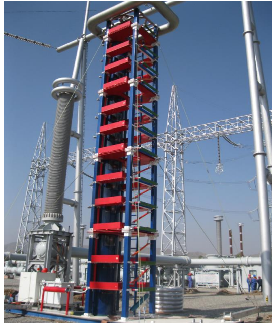
Figure 1. On-going oscillating impulse withstand test implemented on gas insulated switchgear in the field.
