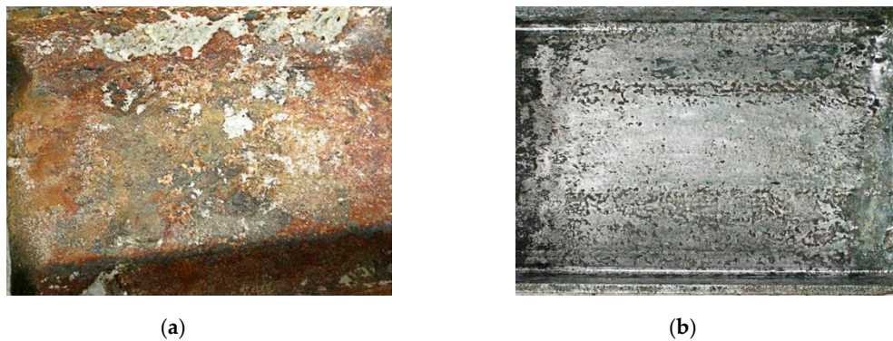
Figure 3. The state of I-shaped steel. (a) I-shaped steel after corrosion; (b) I-shaped steel after corrosion rust removal.
