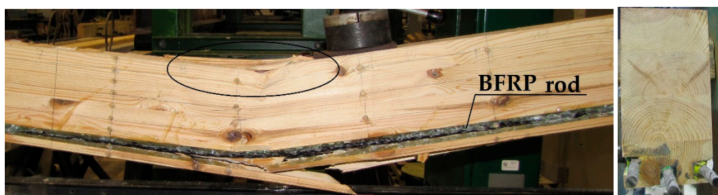
Figure 13. Crushing of the Wa-B1 beam's compressed zone and the destruction of the stretched zone near wood flaws (photograph by Wdowiak).
