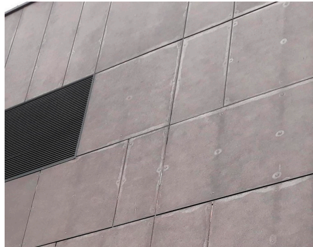
Figure 1. An example of a FCB façade showing considerable damage after ten years of exposure to climate hazards.
