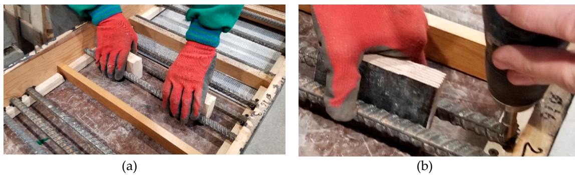
Figure 7. Stabilization of reinforcement in formwork: (a) distance resulting from wooden spacers, (b) rebar fastening to wooden washers with screws.
