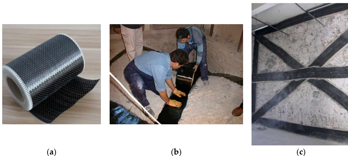
Figure 1. Application of a carbon-fiber-reinforced polymer (CFRP) sheet: (a) a CFRP bi-directional sheet, (b) use of epoxy-resins to bond the CFRP on the masonry surface, and (c) a reinforced wall panel.
