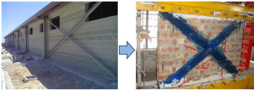
Figure 2. Statics of the resisting mechanism: from a steel structure to a CFRP-reinforced wall [13].
