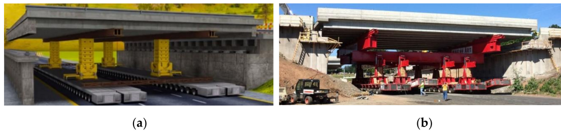
Figure 8. (a) Illustration of placing a new bridge deck with the use of an SPMT (computer-controlled platform vehicles) with jack-ups [19]; (b) placing a bridge with an SPMT during the replacement project, I-84 bridges over Marion Avenue in Southington, US [20].
