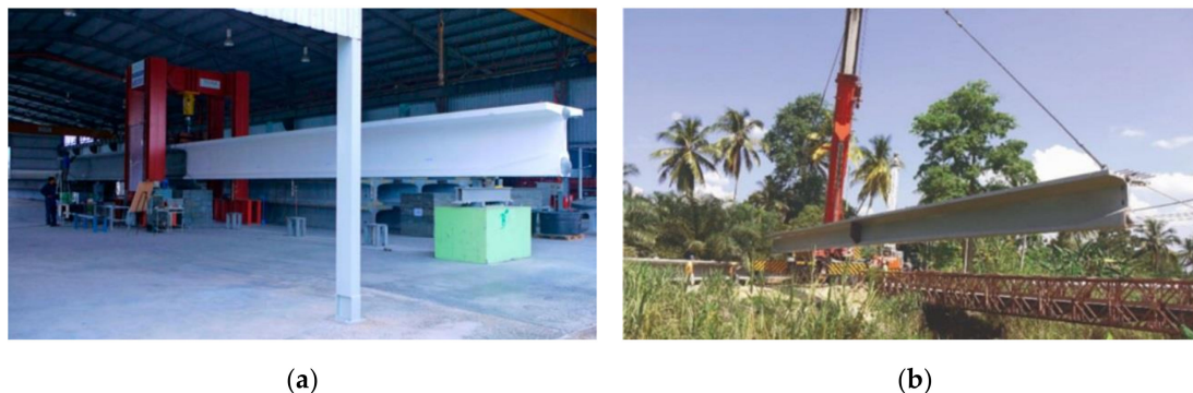
Figure 7. (a) Full-scale destructive test on a 30 m long segmental T-beam, research done in 2007–2010 [14,15]; (b) construction of 30-m-span Ulu Chemor bridge, stitched T-girder construction [15].
