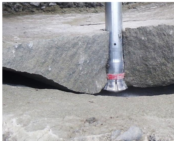
Figure 2. Rock fracture with a single undercut anchor.
