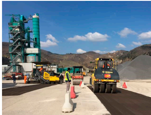
Figure 6. Compaction of CRAM binder course of Subsection C by using the 22-ton pneumatic-tired roller.
