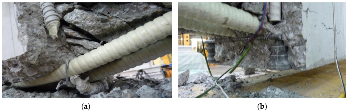
Figure 9. Failure mode of support zones: (a) reinforced with GFRP stirrups; (b) reinforced with GFRP headed bars.
