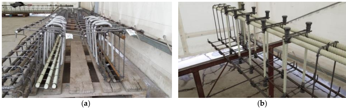
Figure 2. Reinforcement details of test specimens based on example beams: (a) B-1 and B-2; (b) B-3.
