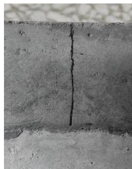
(c) Through crack
