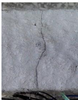
(b) Surface crack
