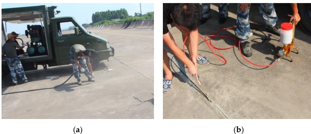
Figure 14. Brief application process. (a) Blowing joints by high pressure air gun. (b) Injecting the PCFC.
