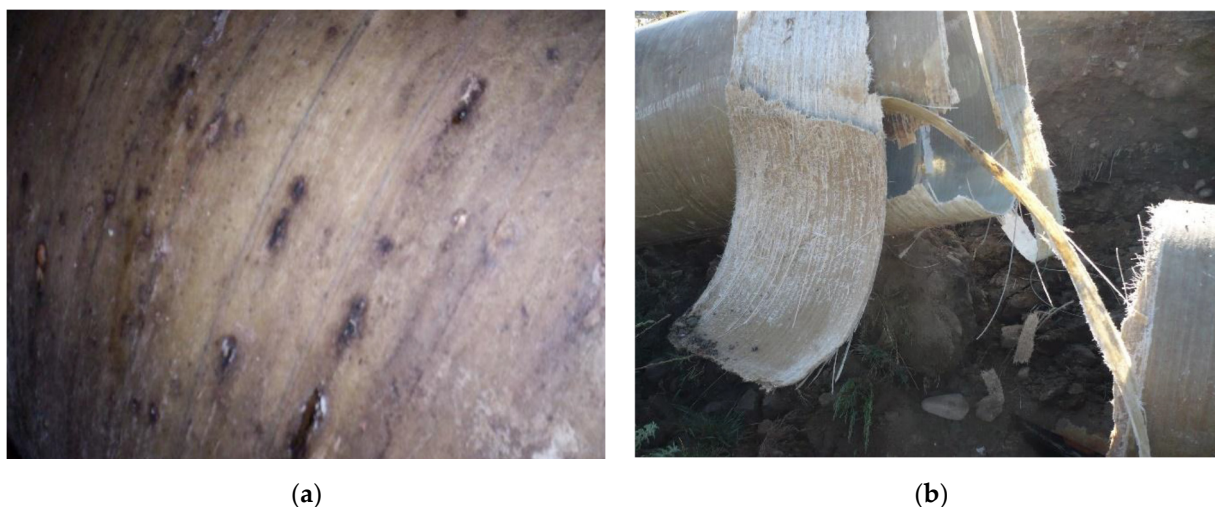
Figure 1. Damage to the glass-reinforced plastic pipeline in (a) basic soil and (b) acidic soil.
