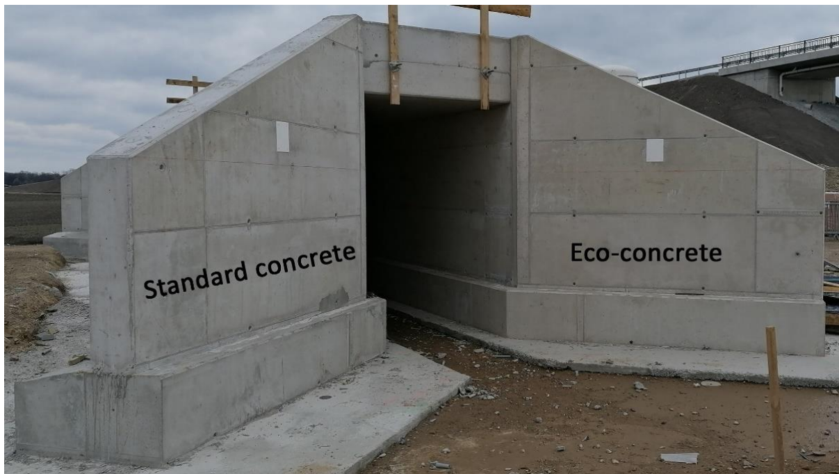
Figure 11. Entrance portal of the small animal subway. The left construction side in standard concrete and the right one in Eco-concrete (© Autischer, IMBT).
