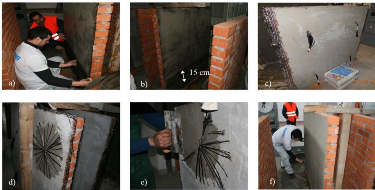
Figure 9. Construction stages: (a) application of the first layer of mortar and reinforcing meshes; (b) overlap of the reinforcing meshes; (c) insertion of composite cords; (d) cords spreading in a circular pattern; (e) embedment of the cords with mortar; (f) surface levelling and final checks.
