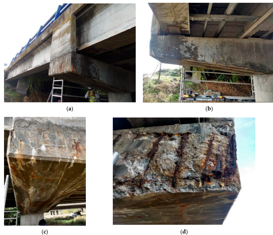
Figure 1. (a,b) Structure analysed from different perspectives; (c,d) Detailing (photos taken by S. Chinchón-Payá).
