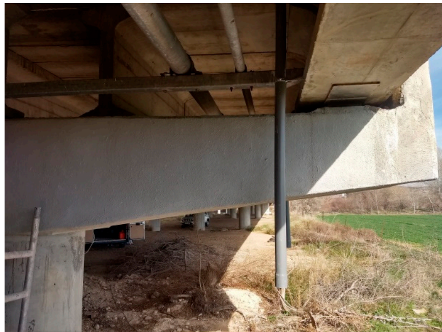
Figure 7. Photograph of concrete member 2 weeks after repair (photo taken by RETINEO).
