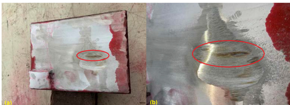
Figure 3. Appearance of the welded plate after liquid penetrate test (a) and cracks (b).
