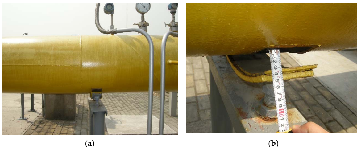
Figure 4. Diagram of pipe breakaway support on the site: (a) general view of the pipe disconnecting bracket; (b) enlarged view of the pipe disconnecting bracket.
