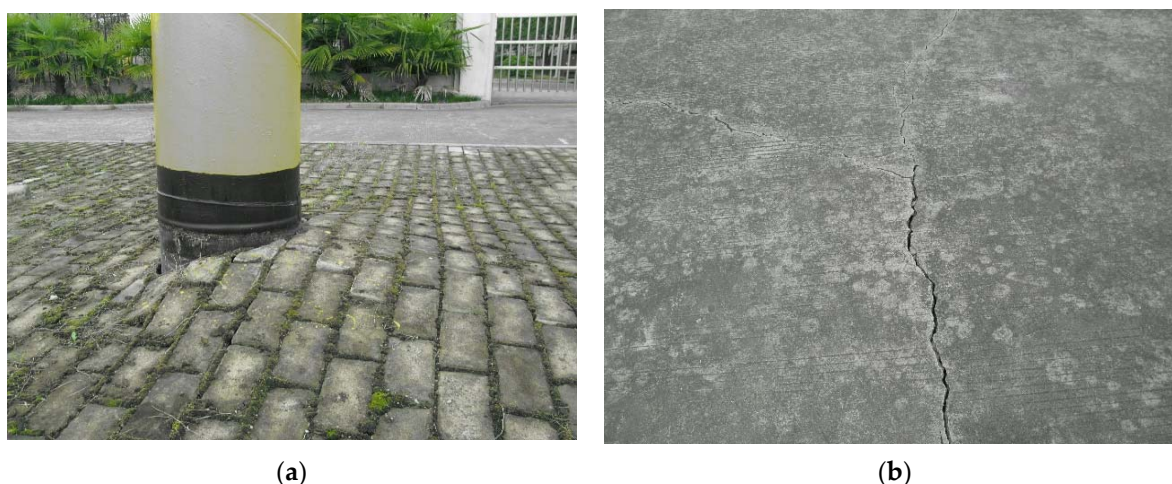
Figure 3. Ground conditions on the site: (a) the ground heaved at the pipeline into the ground I; (b) the ground heaved and cracked at the buried pipe.
