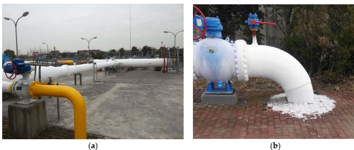
Figure 2. Frosting of pipes on the site: (a) frosting of the above-ground pipeline; (b) frosting of the pipeline into the ground.
