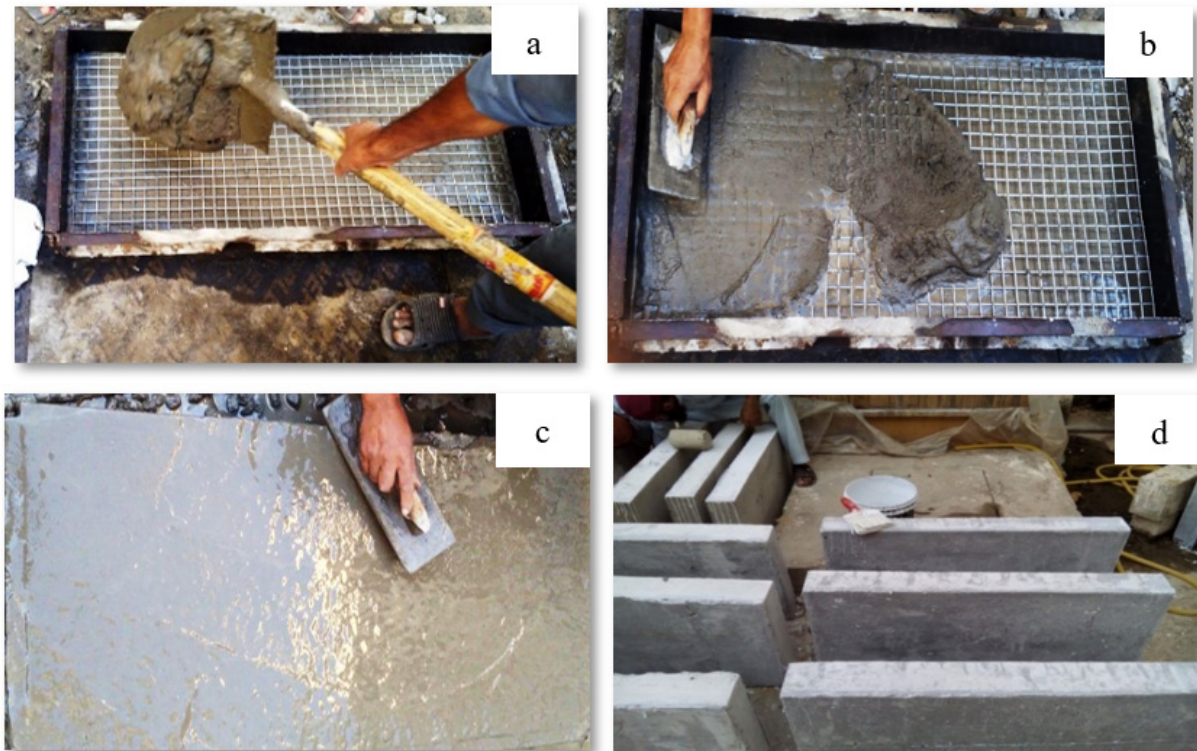
Figure 6. (a) Placing of ferrocement mesh and mortar; (b) Spreading of mortar over the mesh with a trowel; (c) Final finish with a trowel; (d) Whitewash on sides of slabs.
