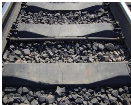
Figure 16. Track bed hardening damages the concrete sleeper.
