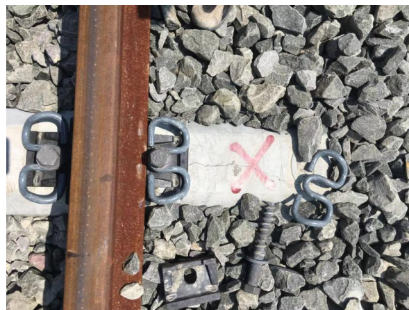
Figure 14. Excessive torque of the buckling bolt causes sleeper damage. Note: These images also show other factors in addition to the torque of the buckling bolt.
