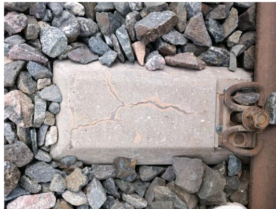
Figure 11. AAR damaged the concrete sleeper. Note: These images also show other factors in addition to AAR.
