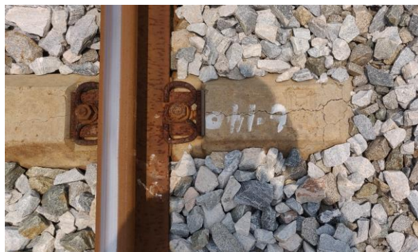
Figure 12. DEF damaged the concrete sleeper. Note: These images also show other factors in addition to DEF.
