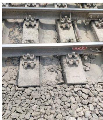
Figure 17. Track bed frost boiling damages the concrete sleeper.
