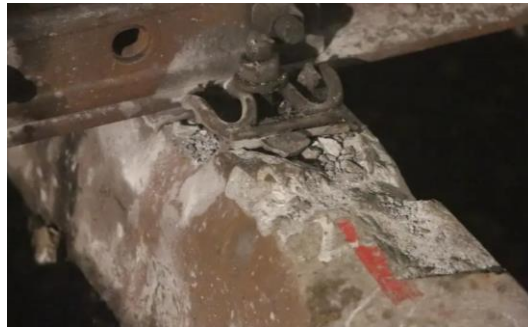
Figure 13. Damaged concrete sleeper in the derailment.
