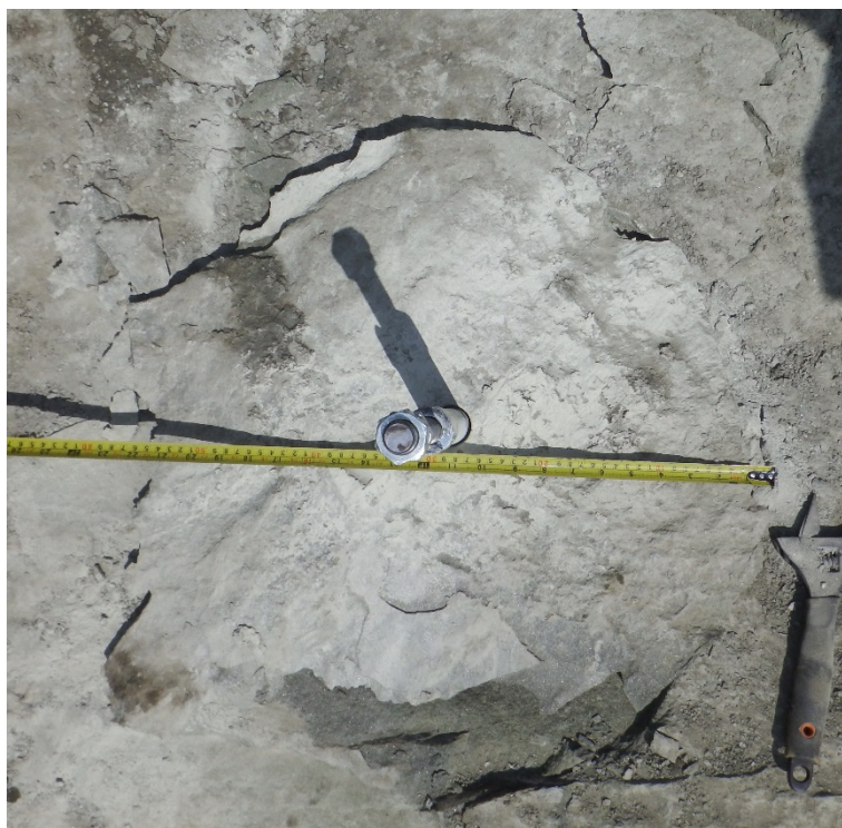
Figure 10. Measurement of the extent of the failure cone on the free surface of the base rock material.
