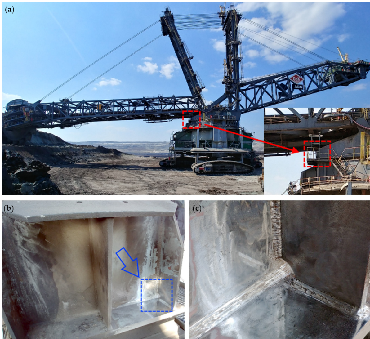
Figure 7. Structure under investigation: (a) general view; (b) the joint; (c) research area.
