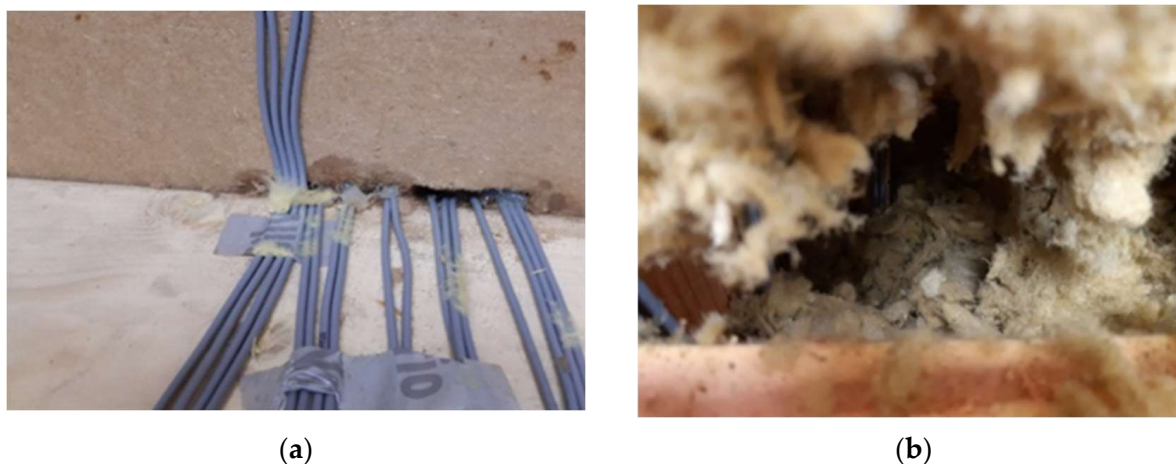
Figure 8. Detected defects: (a) Increased moisture transfer in fragment E3; (b) Air cavity in the middle of S2.
