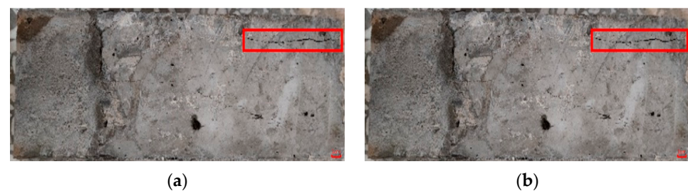
Figure 12. Partial cracking damage status of the OC/ECC slant shear test specimens. (a) OC/ECC-N; (b) OC/ECC-Y.
