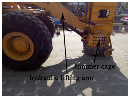
Figure 1. Micro-crack homogenization crushing of pavement structure [2].
