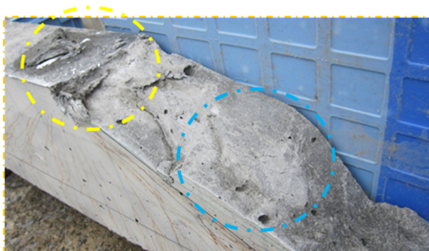
Figure 4. Fracture surface of the SHCC member and normal concrete.
