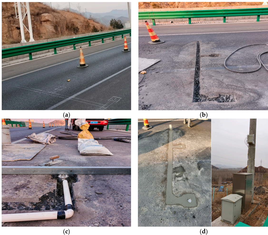
Figure 5. Installation of sensors in Laiqu Expressway in Hebei Province, China: (a) preparation of safety work; (b) grooving of pavement; (c) installation of the sensor; (d) rehabilitation of pavement and establishment of data transmission pathways.
