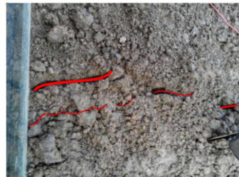
Figure 9. Cracks on sides of the slope (Test 3).
