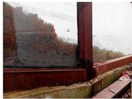
Figure 8. Vertical crack at the back edge of the slope (Test 1).
