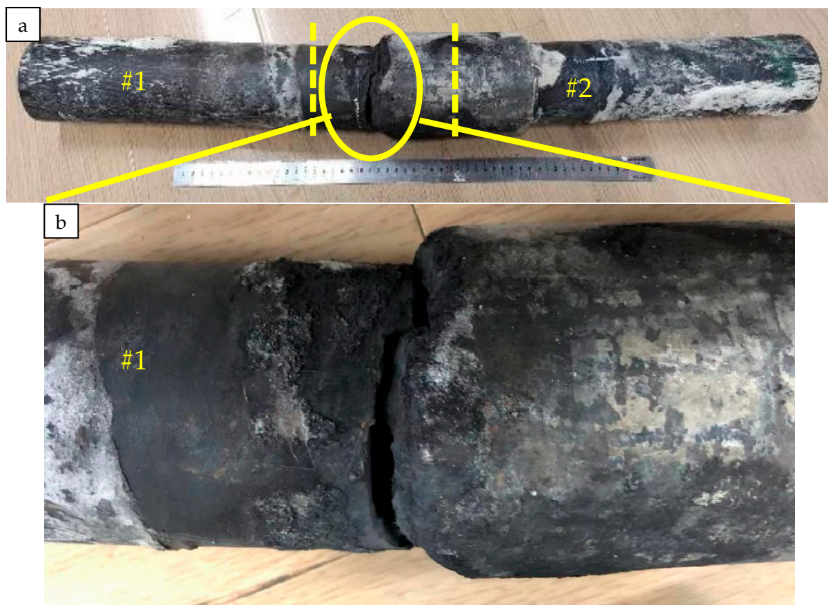
Figure 1. Macroscopic morphology of failed pipe section. (a) The whole pipe (b) The cracked section.
