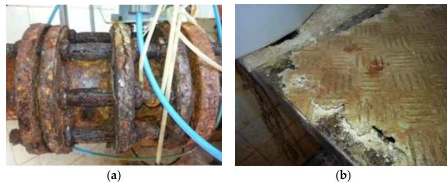
Figure A1. Joint screws on the reservoir water inlet pipe (a) and reservoir floor (b) uniform corrosion and in the form of cracks in the municipal facilities.
