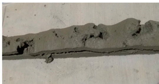
Figure 1. Defect in the printed foam concrete.
