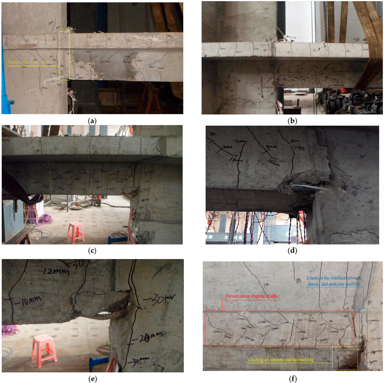
Figure 12. Typical damage of specimens. (a) Crack distribution of JD1. (b) Crack distribution of JD2. (c) Crack distribution of JD3. (d) Crushing of concrete. (e) Bar buckling. (f) Flexure–shear diagonal cracks and cracks at the interface between precast and post-cast concrete.
