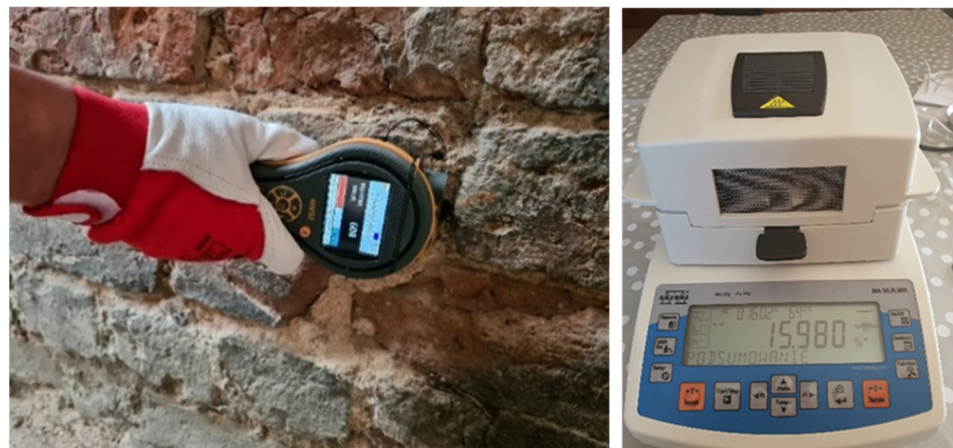
Figure 8. Assessment of the moisture level of walls using the radio and laboratory dry-oven test method (photos by the authors).
