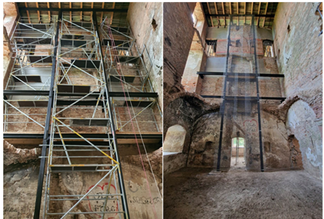
Figure 14. Current view of the strengthened wall and the strengthening structure (photos by authors).
