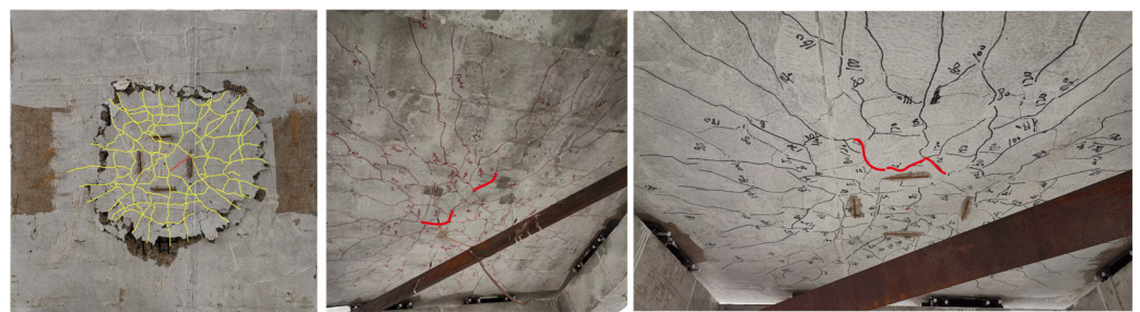
Figure 7. Distribution of cracks on the bottom surface of the slab. Red line indicated the first crack; yellow line indicated the distribution cracks after punching shear.
