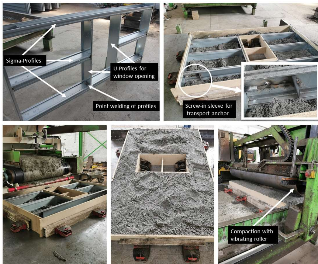
Figure 2. Manufacturing process of prototype at precast plant. ( Top left ) framework of steel profiles, rotated by 90°; ( Top right ) Partial filling of the formwork with LAC+; ( Bottom ) Filling and compacting of the wall element.
