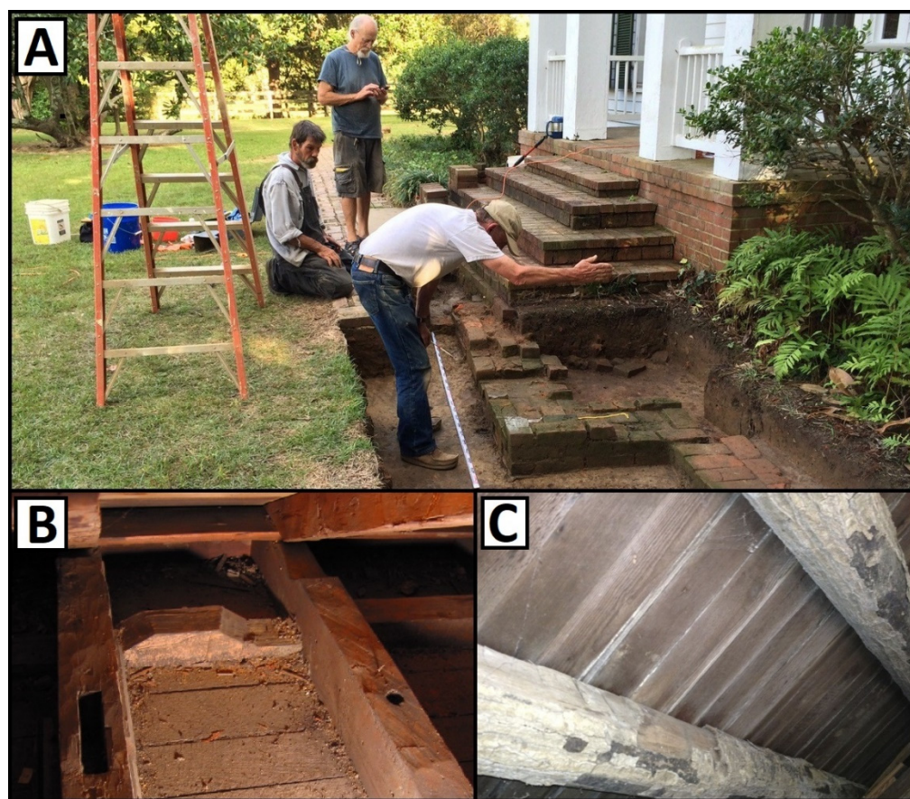
Figure 1. Walker House (A) pre-existing brick foundation, (B) hand-finished attic timbers, and (C) crawlspace oak joists. Photos by R. Doherty.
