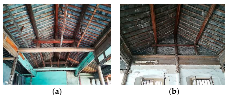
Figure 2. Structure types; (a) post and lintel construction frame; (b) column and tie construction frame.
