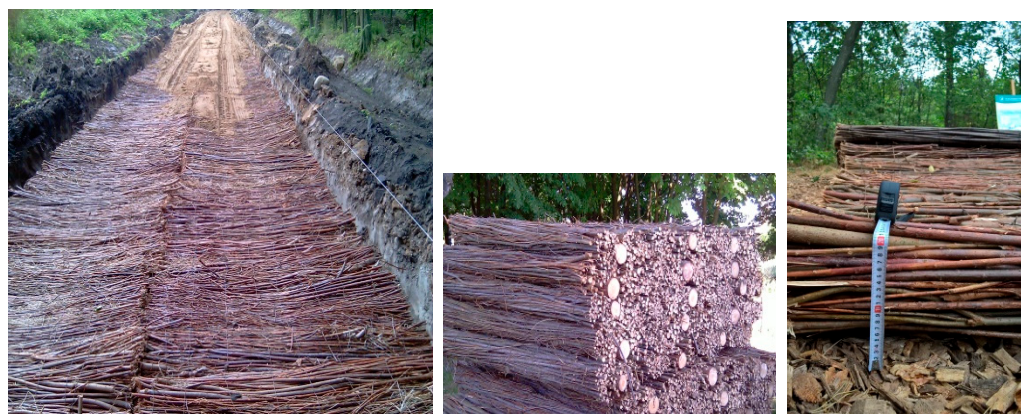
Figure 2. Reinforcement of the roadbed in the studied sections—willow brushwood mattress with and without logs reinforcements built in trial.
