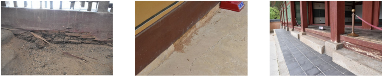
Figure 2. Types of contact between the ground and wooden items in wooden cultural buildings in Korea.
