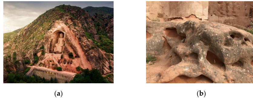
Figure 14. (a) Buddha statue in Cave 5; (b) wind erosion symptoms of Buddha foot.
