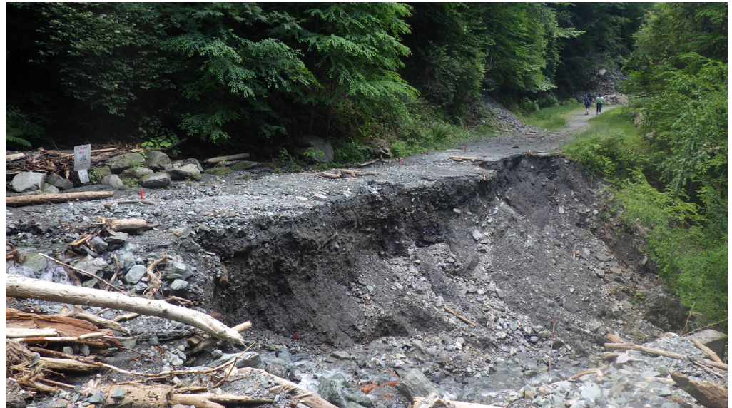
Figure 1. Image of forest road failure. A culvert at a stream crossing was destroyed by heavy rain, and the road body was eroded by stream water, making it inaccessible to vehicles.
