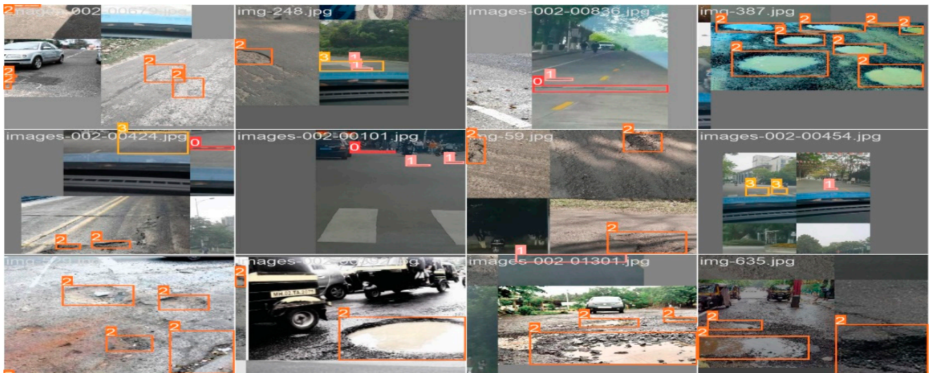
Figure 1. Complex types of road surface defects. 0 is the speed bump, 1 is the manhole cover, 2 is the pothole, and 3 is the fracture.
