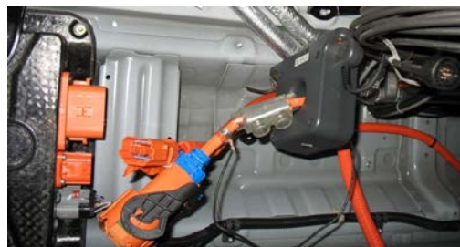
Figure 7: Picture of the disconnected high-voltage battery main cable with a high current fuse looped through a 500A solid-core amp probe
