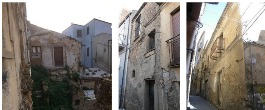
Figure 2. Examples of abandoned and partially collapsed buildings in the historical centre of Enna.
