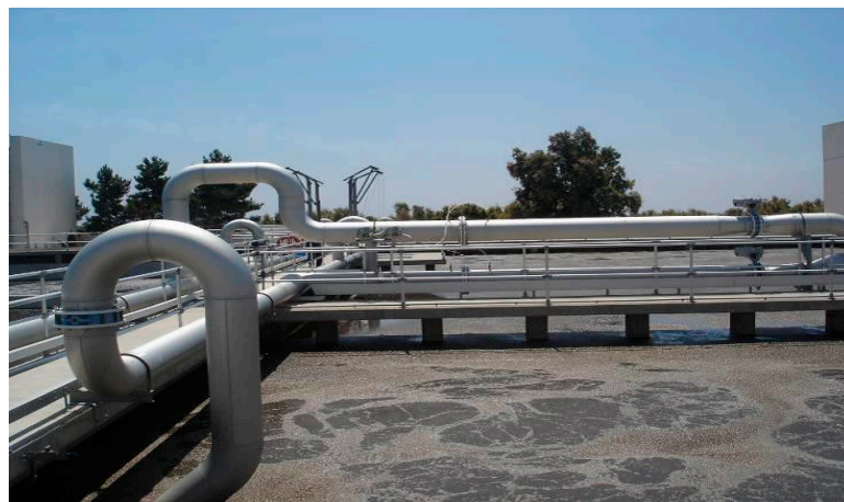
Figure 6. Biological reactor with air distribution network.
