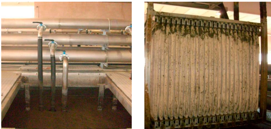
Figure 7. Membrane cassette with aeration and permeation ducts.
